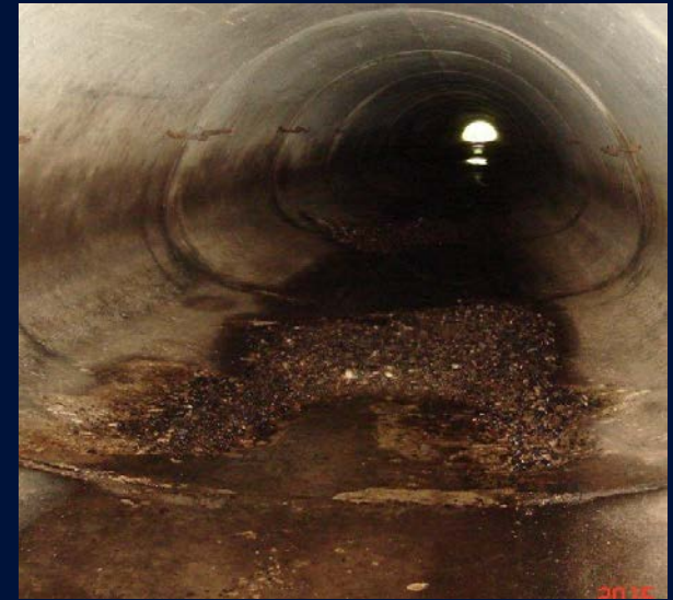
Bad concrete mix in alternating pipe sections, District 3 Baxter
