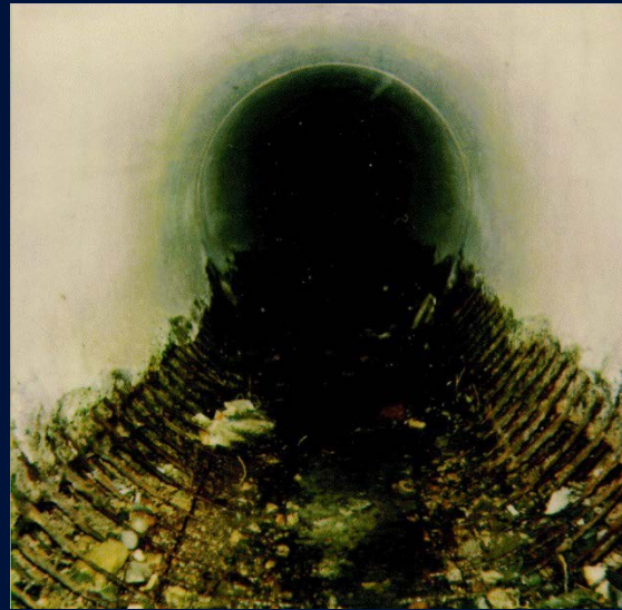
Acidic factory discharge, I-94 St. Paul Metro District
